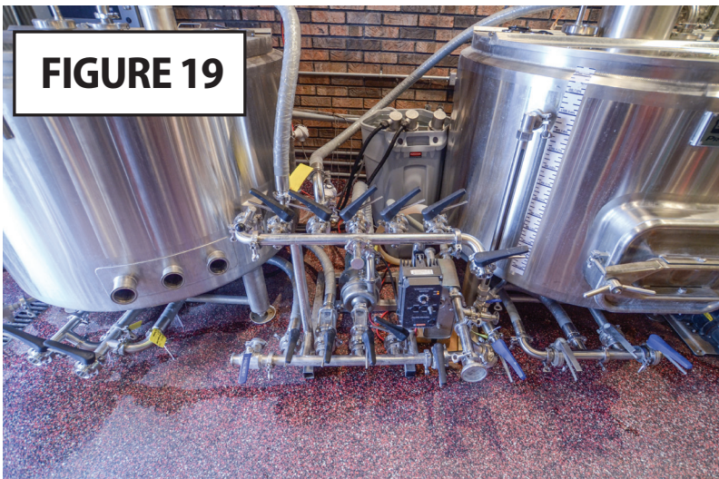
Straight view of the manifold assembled.
