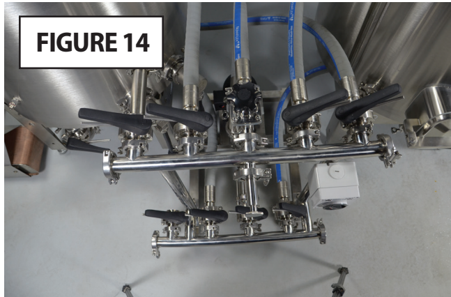
Top view of manifold.
