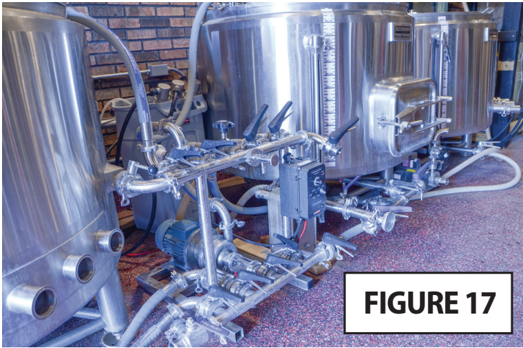
Side view of the manifold assembled.
